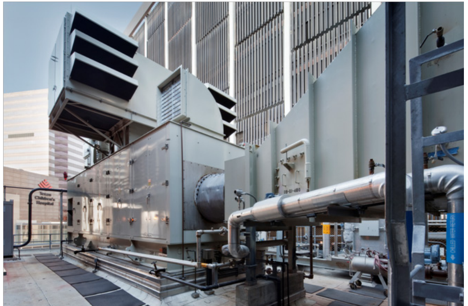
The gas turbine-based CHP system at Houston Methodist Hospital improves the hospital's energy security and reliability and eliminates the need for a diesel back-up generator
