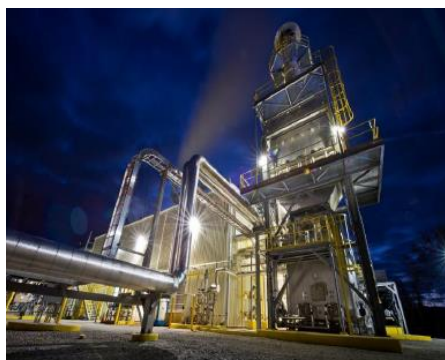
DTE Marietta CHP Plant at Solvay Specialty Polymers (Source: DTE Energy)
