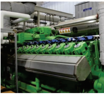
A 1.4 MW engine installed in 2015 at the Des Moines Wastewater Treatment Plant followed streamlined air permitting procedures.
