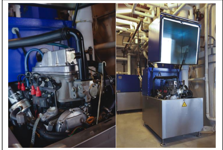
One of two 19 kW EC Power (Lochinvar) XRGI® Natural Gas-Fueled Reciprocating Engines and Engine in Sound-Proof Enclosure
