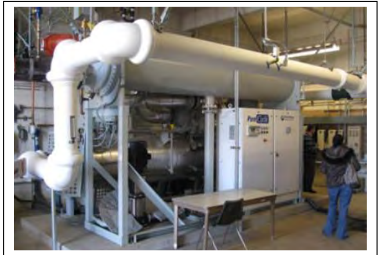
280 kW binary Pratt & Whitney PureCycle ORC powerplant at OIT (Geo-Heat Center)
