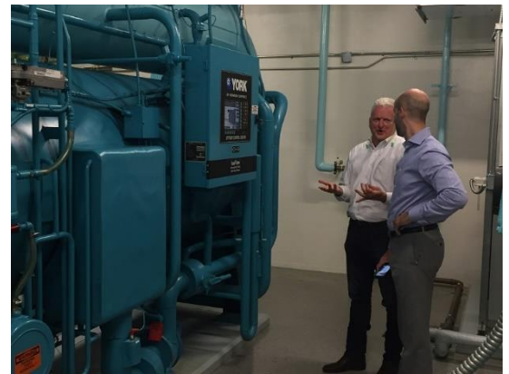
York Absorption Chiller
