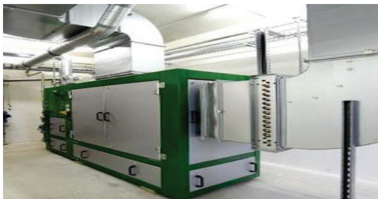
Small Modular CHP Unit < 10 MW
