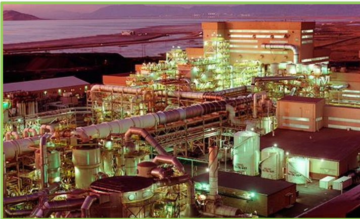
Kennecott Utah Copper Smelter Salt Lake City, Utah 32 MW Waste-Heat-to-Power CHP System
