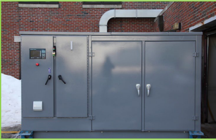
A 150 kW CHP system prior to installation at St. Mary's d'Youville Pavilion, a non-profit nursing home
