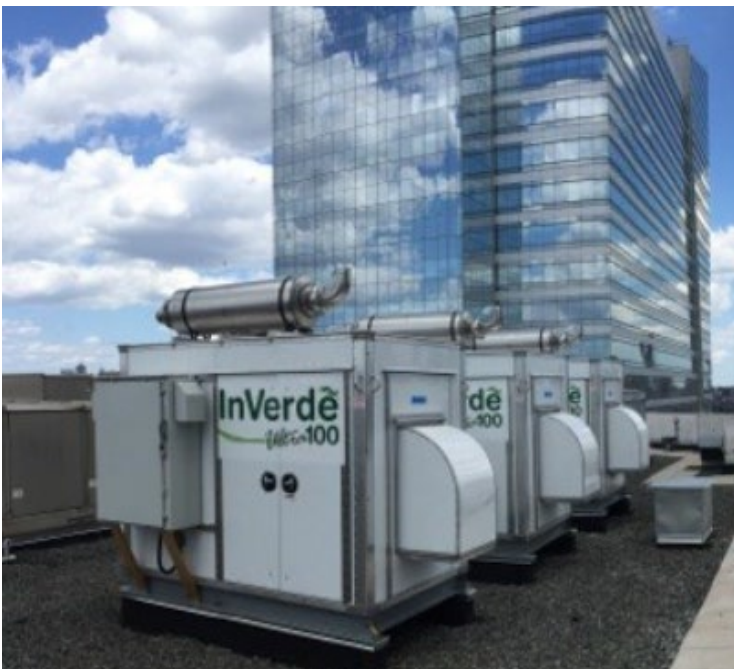
A 300 kW Tecogen CHP system installed at the Westin Jersey City Newport
