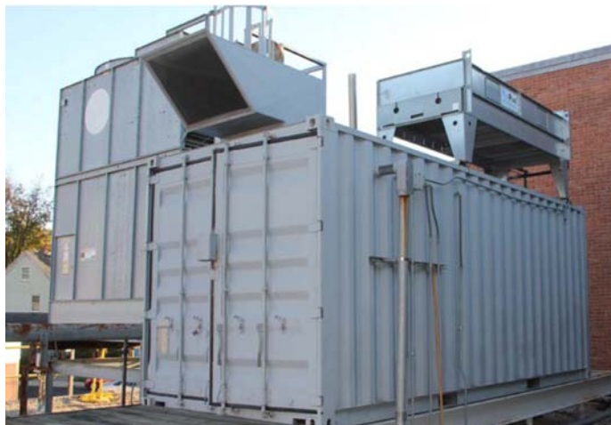
The 335kW CHP systems is housed in two separate containers. The first to be installed was the 250kW AMERIGEN8250, followed by the 85kW AMERIGEN8085
