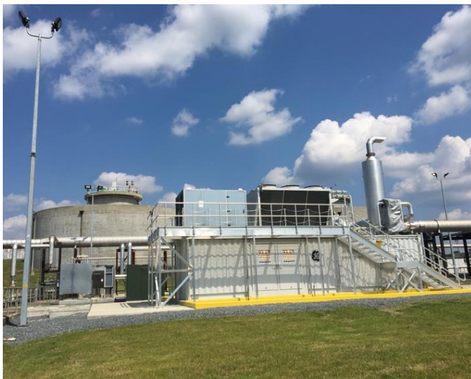
Biogas CHP at McAlpine WWTP in Pineville
