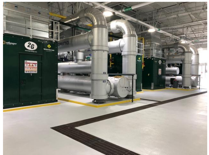
Each pair of gensets at Erlanger Hospital is connected to one heat recovery steam generator (2 HRSGs total) to optimize steam generation. PHOTO COURTESY OF 2G Energy
