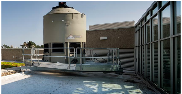
The CHP system at Washtenaw Community College reduces the college's carbon footprint.
