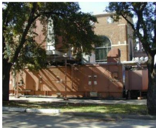
Rice University CHP plant.
