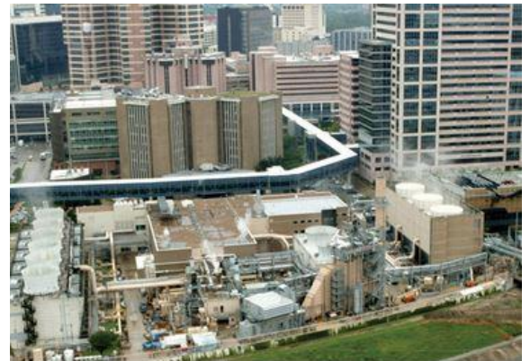
TECO district energy plant.
