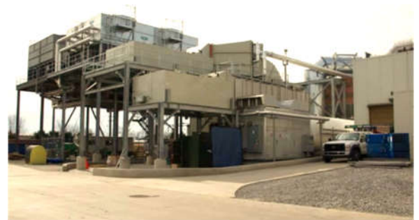
H.P. Hood CHP Plant in Winchester, Virginia (15 MW combustion turbine CHP plant)
