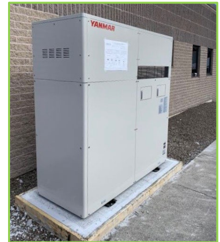
One of two 35 kW Yanmar reciprocating engines
