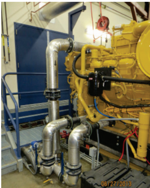
Diesel engine with attached heat recovery system at the Point Lay Powerhouse in Alaska's North Slope Borough.
