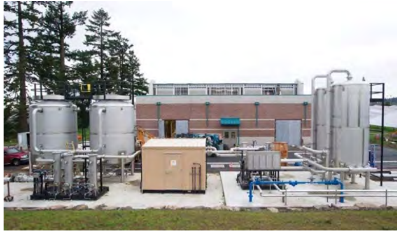
A Unison Solutions gas conditioning system is located outside of the cogeneration building.
