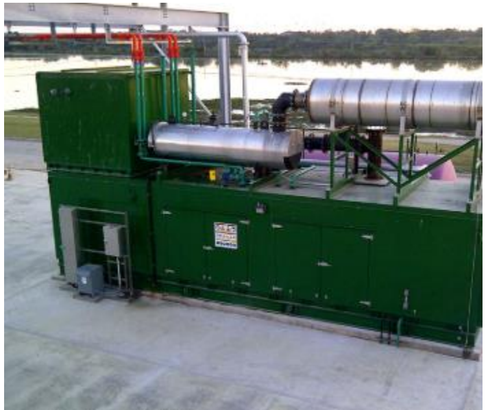
850 kW Reciprocating Engine
